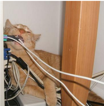
At Risk of Electrocution
